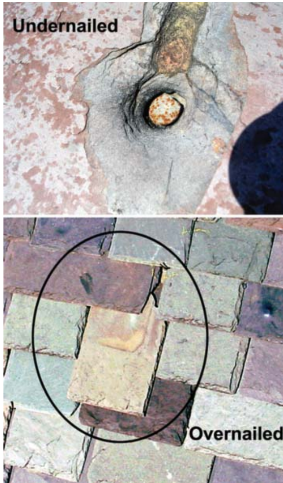
Figure 15: Under-nailed slates aren't driven in far enough, leaving a protruding nail head to rub against the overlying slate, eventually to wear a hole in it. Over-nailed slates become broken when the nail is driven through the slate. [Photos by Joseph Jenkins]
