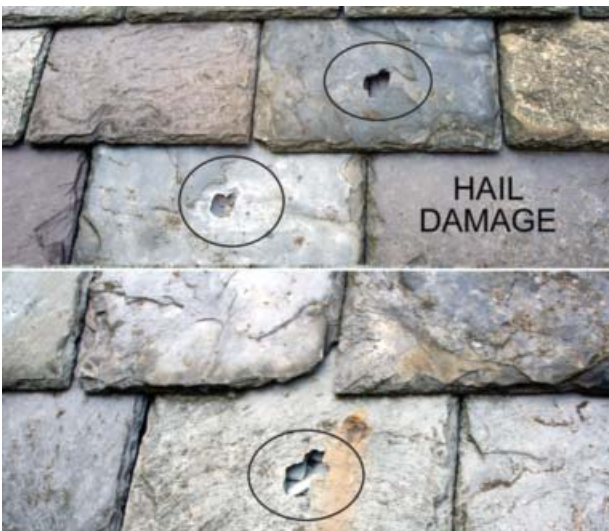
Figure 16: External punctures, such as from large hail stones, leave holes with sharp edges, as shown here. The crater is always opposite the impact side. [Photo by Joseph Jenkins]
